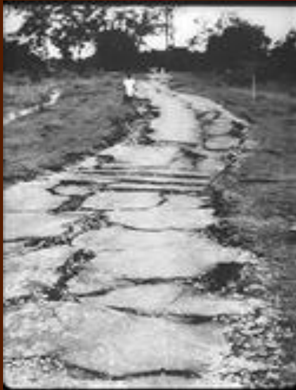
Cracks in the Assam Trunk Road (Khowang?), N.E. India KVS
